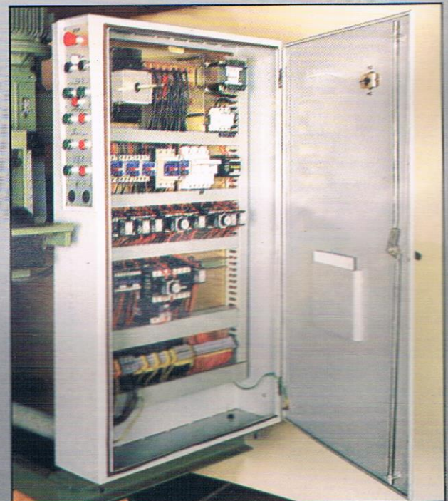
– Control panel and main electrical entrance
